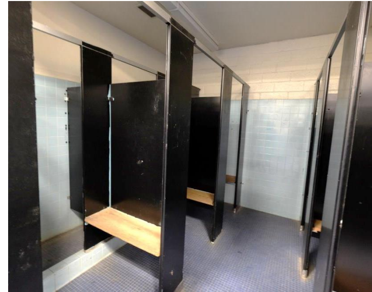
Photo 19 Building Name: Shower/Locker Building Number: 3 Private showers that generally are not used.
