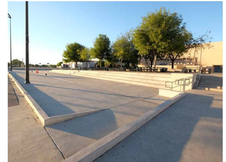
Photo -5 Stairs to lower athletics do not appear to comply with accessibility standards.
