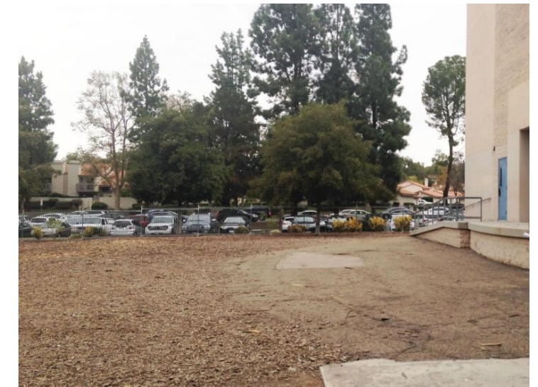
Photo -1 Pavement to ramp access in need of repair.
